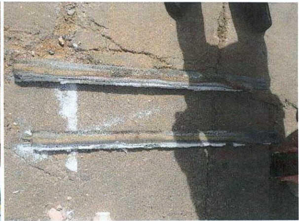
Photo A3-17 View of the joint material removed (top: joint 2, bottom: joint 1)
