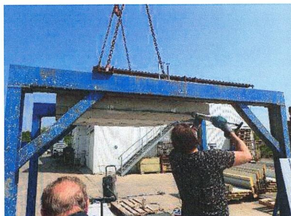
Photo A3-5 Sealing the panel edges with Tendonol® Fire Protection Sealing Compound
