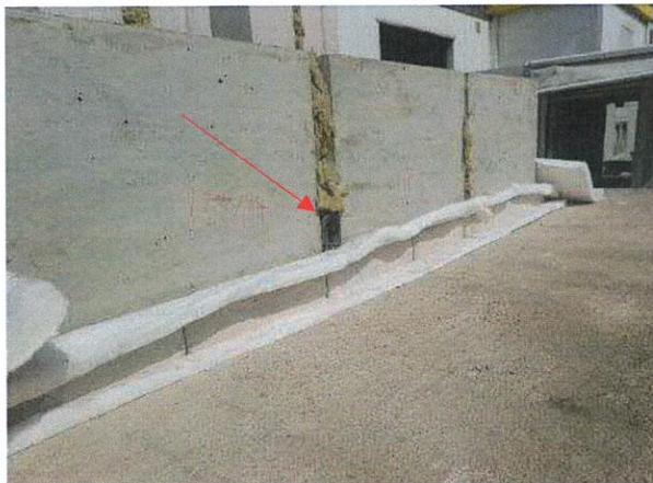
Photo A3-12 Slight brownish discolouration at joint 2 – 106th minute
