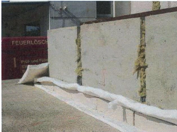
Photo A3-10 Some smoke escapes from joint 2 – 36th minute
