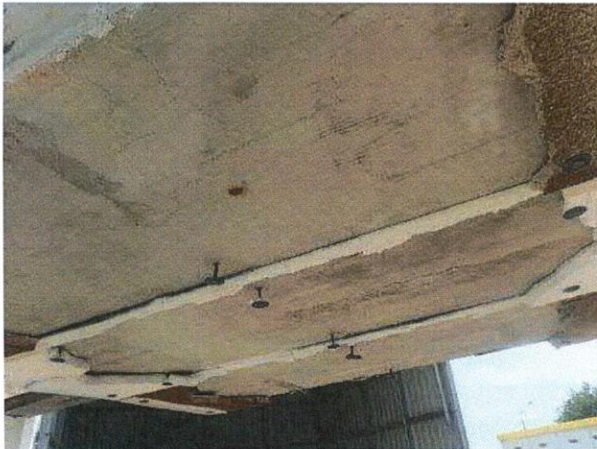
Photo A3-16 View of the joint material used (fire protectional panels were removed manually)
